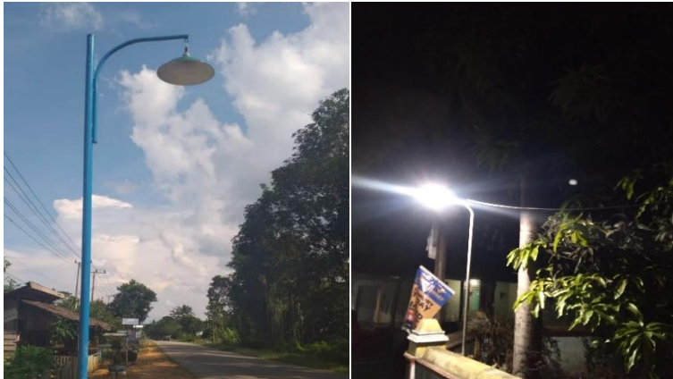
Figure 1. Conventional lamps in Andongsili Village
