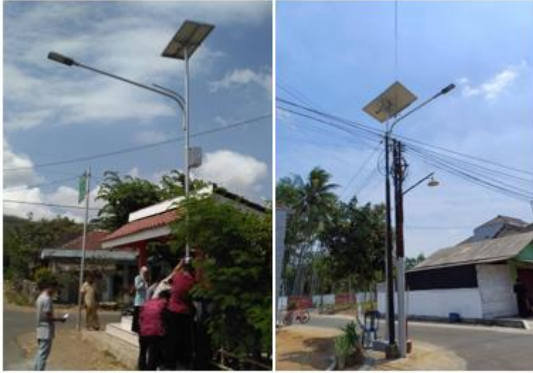
Figure 2. Solar Panel Street Lights (PLTS) in Bumerto Village
